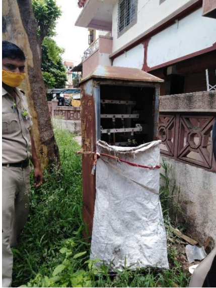
Figure 6: Open feeder pillar box 1
