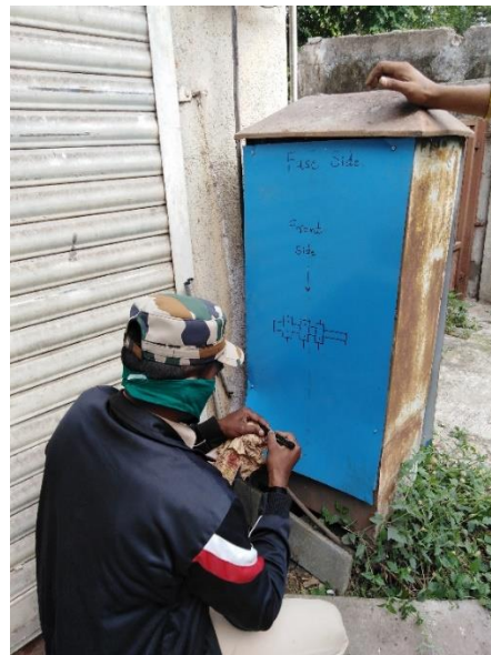
Figure 9: Markings for easy understanding of fuse side of feeder pillar
