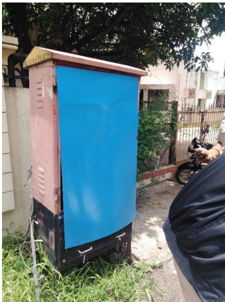
Figure 8: Sheet used to close feeder pillar
