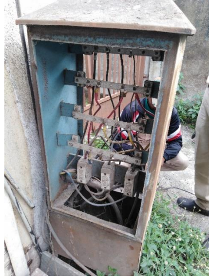
Figure 7: Open feeder pillar box 2
