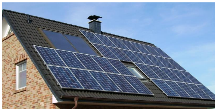
A rooftop with solar cells.
